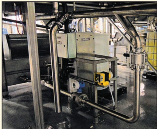
The compact size of the BioIonix system allows it to fit into tight spaces. As shown in the photo, the reactor module is below the mezzanine that contains the vegetable washing flumes, while the BioIonix power and control cabinet is located on the mezzanine itself for operator convenience.
